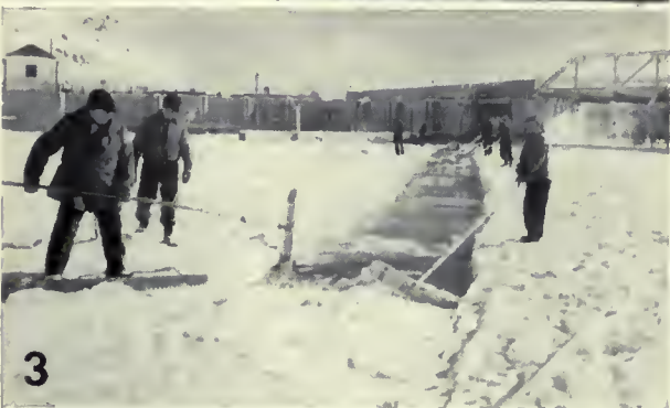
HEADING OFF THE SLUSH FROM THE HEADGATE.— (1) Wind River Diversion Dam and headgate of the Wyoming Canal, with dotted line indicating the location of the by-pass channel when the water back of the dam freezes solid; (2) and (3), opening a channel in the ice behind the dam to carry the slush ice through the log-way, and thereby divert it from the headgate of the canal which feeds water to the Pilot Butte Power Plant. Temperature—25 degrees below zero.
